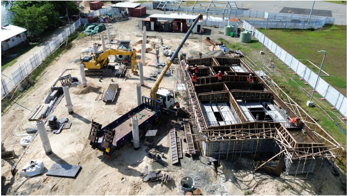
Photo 3 - The use of new types of heavy machinery on locally delivered projects provide training and skill development for the 100 percent local workforce.
