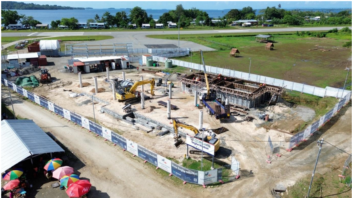
Photo 4 - The new Seghe Market will provide space for up to 120 vendors with shower and toilet facilities for men, women and people with disabilities.
