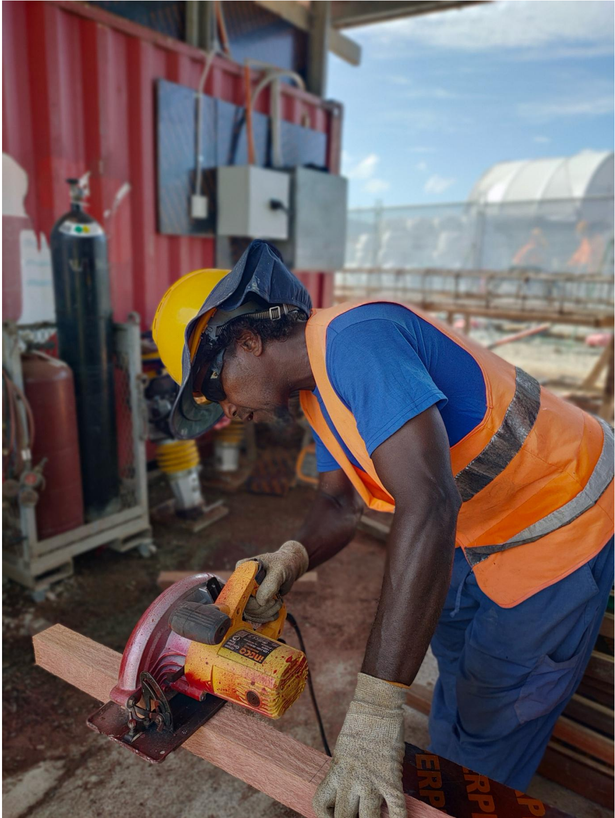
Photo 2: Construction Supervisor, Tagila Hiti, said the project had a good story to tell about improving the skills and knowledge of local workers.
